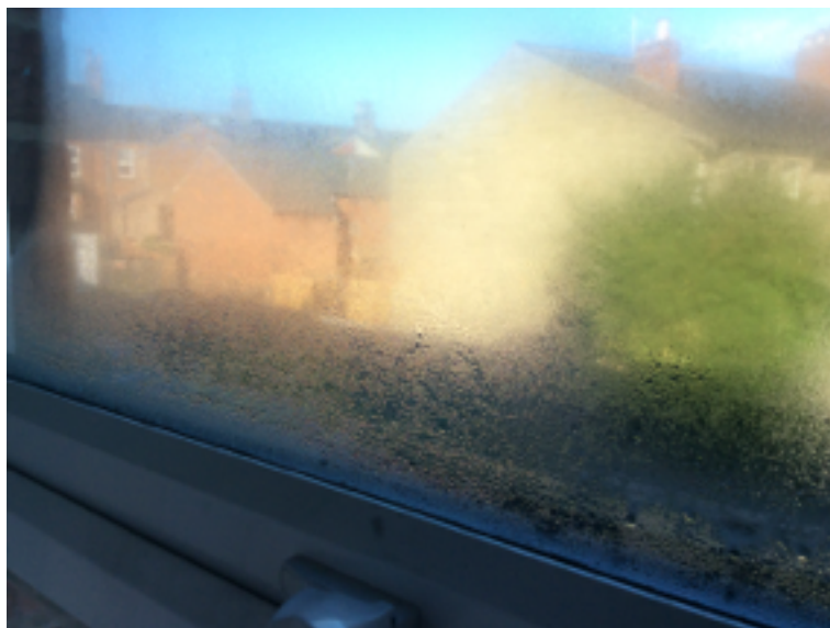
Condensation can form when a room is not properly ventilated.
