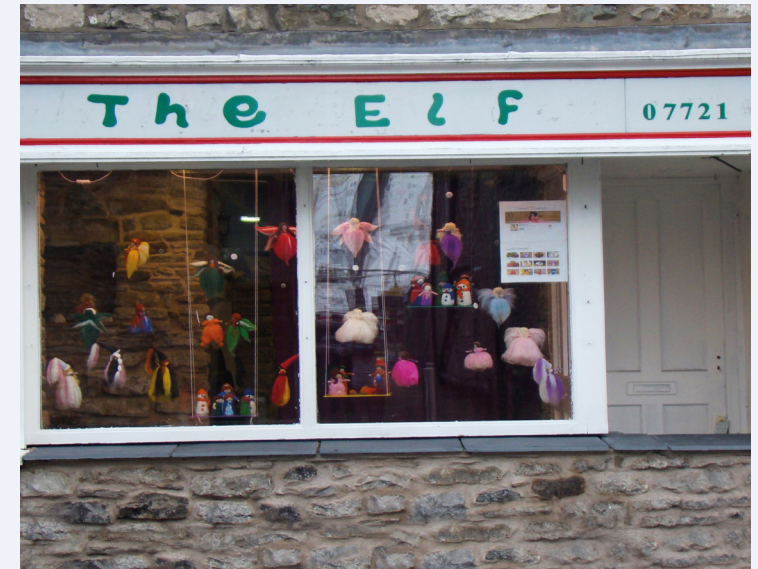
Figure 3 Shop front, with new flood wall to deflect 'bow waves' caused by passing vehicles
