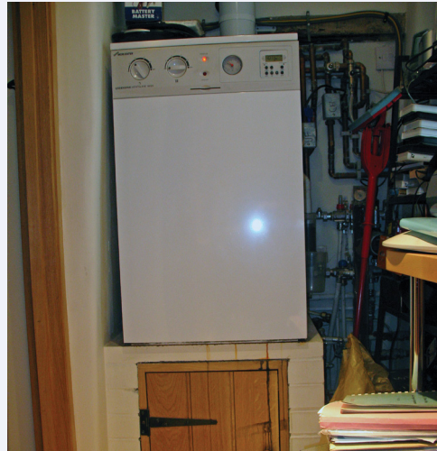
Figure 4 Boiler on plinth
