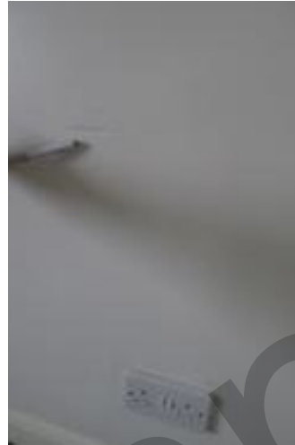
Dent approx 10cm to wall above right double socket on the wall opposite the fitted wardrobes
